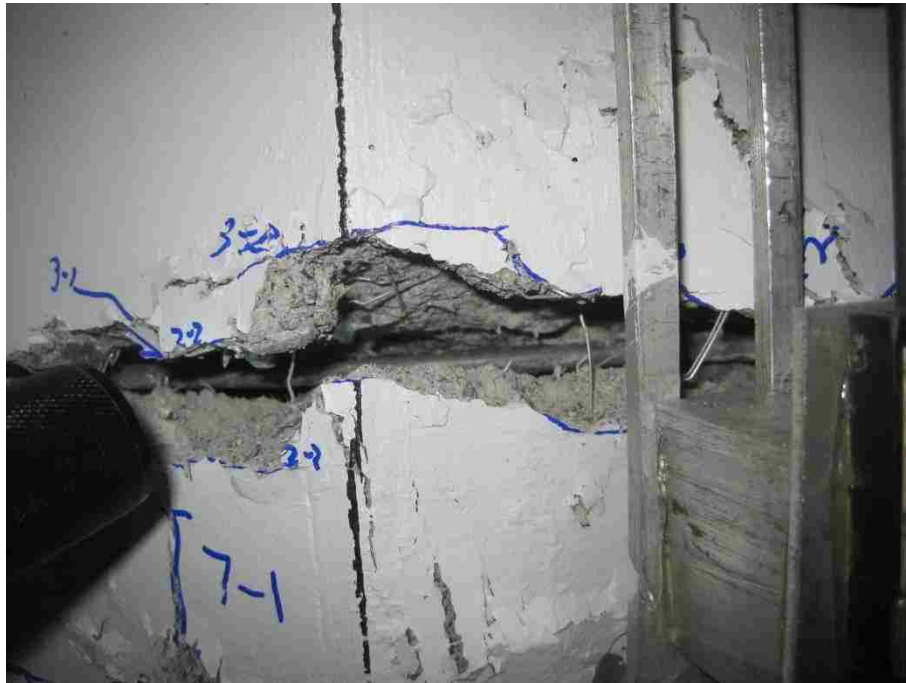
Figure C - 11: Large crack in concrete core, cycle 8-2.
