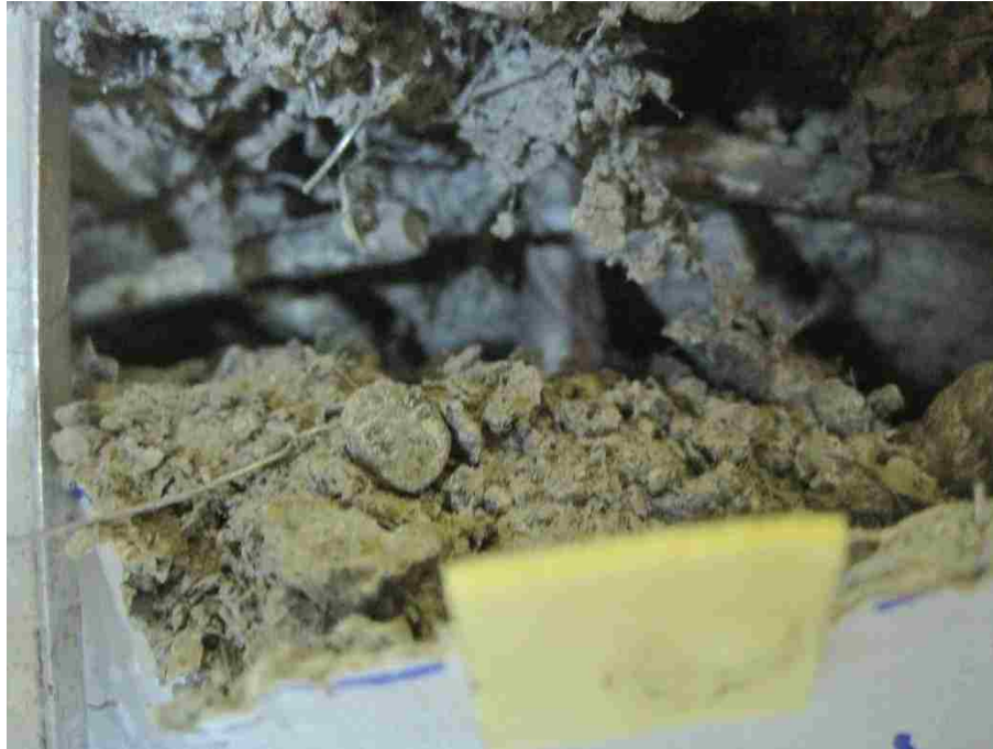
Figure C - 12: Fracture of longitudinal reinforcement bar, cycle 9-2.
