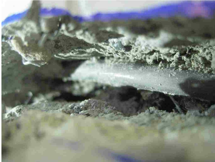
Figure C - 4: Large crack in concrete core, cycle 9-1.
