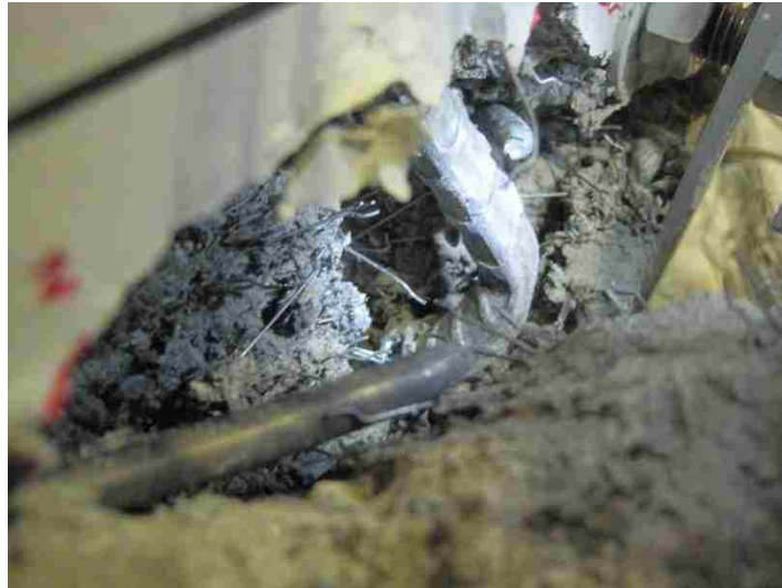
Figure 4-9: PreT-SS buckled rebar and broken spiral.
