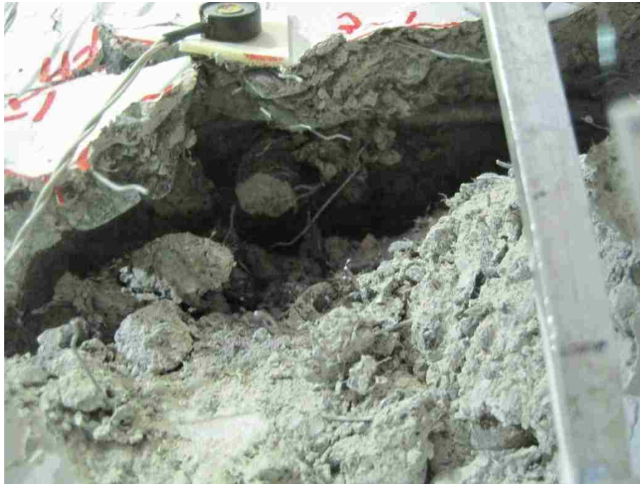
Figure C - 5: Fracture of longitudinal reinforcement, cycle 8-1.
