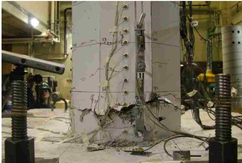
Figure 4-6: PreT-BS fully spalled.
