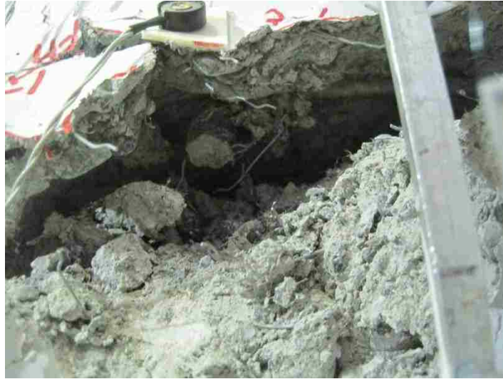
Figure 4-8: PreT-BS broken longitudinal rebar.
